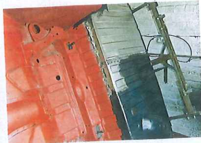
6) APRIL 2013 Yet more welding, as Ian fashions a huge repair panel for the boot floor.
